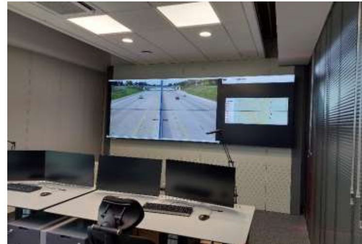
Room of National Road Hotline
